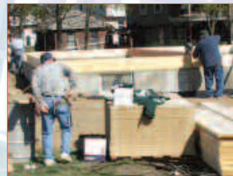
Jack McPike and Mike Mazur of Kennedy Valve donate their time to build the Habitat home.
